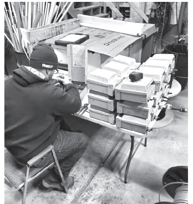
Ryan Dubie of Tandem Electric rewires each light pole receptacle in preparation for hanging lighted Christmas decorations in the Village of Fruitport
